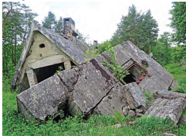
Remains of a bunker house – note the hinges for armoured shutters and fortified chimney. Photo Clive Penfold
